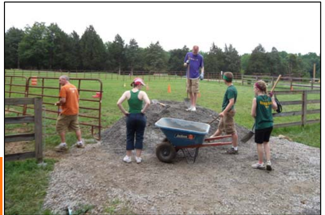
A group of high school youth laying gravel and digging trenches for the roads and water lines at Cedar Ridge Camp in Louisville, Kentucky.
