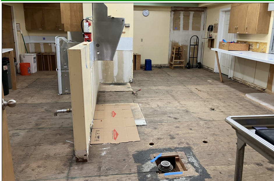
All the appliances and lower cabinets were removed in the upstairs kitchen due to the water damage from the recent ice storm.
